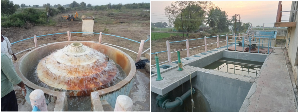
Water treatment and filtration plant at Mandve
