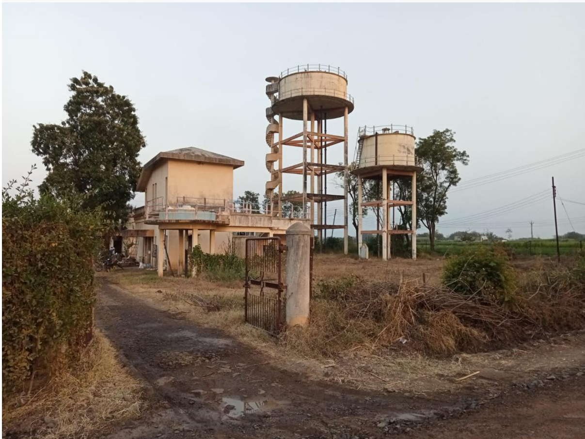
Water treatment and storage facility at Mandve serving eight villages
